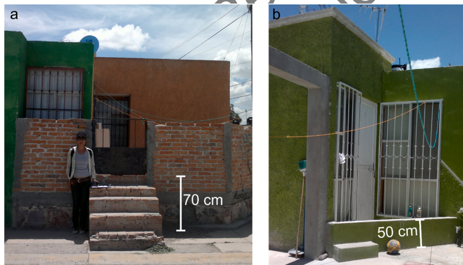
Fig. 7. Examples of modifications in houses to deal with flash floods.
